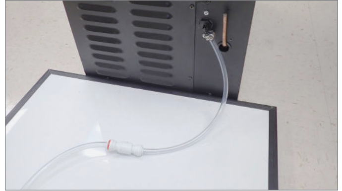
FIG. 6. Installed check valve.
