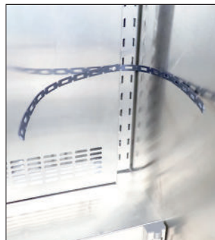
FIG. 8. Installed safety strap.
