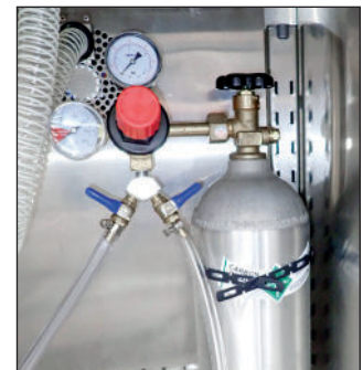
Fig. 9. Always strap the CO 2 cylinder into the cabinet.
